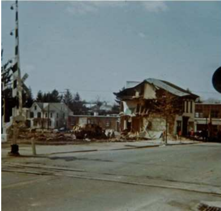
Demolition of flood damaged buildings; Busser's and our shop are already gone.
