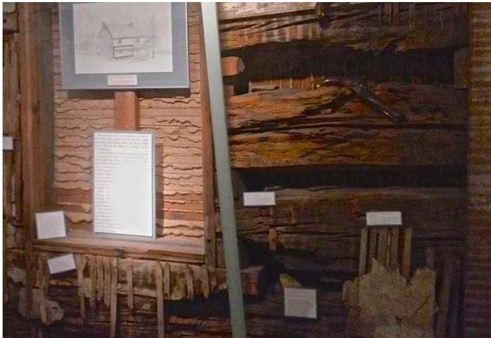
This log wall was discovered while some repairs were being done in the Packwood House Museum in the 1980s. The logs are part of the original log tavern built at the corner of Market and Water streets by about 1800.
