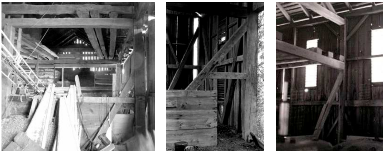
Figure 13 Development of barn frame construction in Buffalo Valley. a) four-bay barn which combines log crib hay mows with a frame bent between the two center bays. Note large opening in the log wall for loading hay into the mow, and overhead moveable beams for additional mow space. b) early four-bay frame barn with all hewn members. Note use of vertical studs at the exterior wall, indicating that the original barn cladding was split horizontal clapboards, later replaced with sawn vertical board siding. c) mid-19 th century five-bay frame barn with mostly mill-sawn frame members. Note horizontal rails at the exterior wall for sawn vertical board siding. All three barns have the large diagonal down-brace typical of framing bents in Buffalo Valley.
